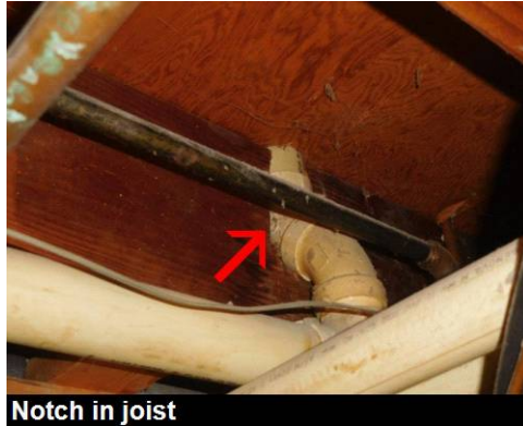
Notch in joist
