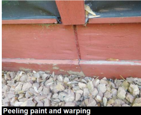
Peeling paint and warping
