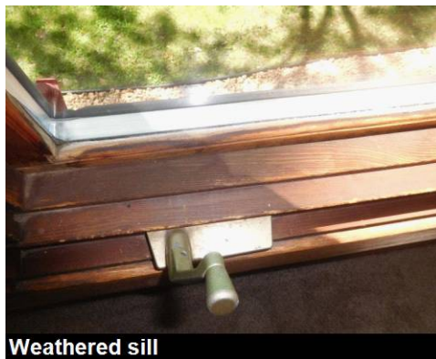
Example of: moisture between panes
