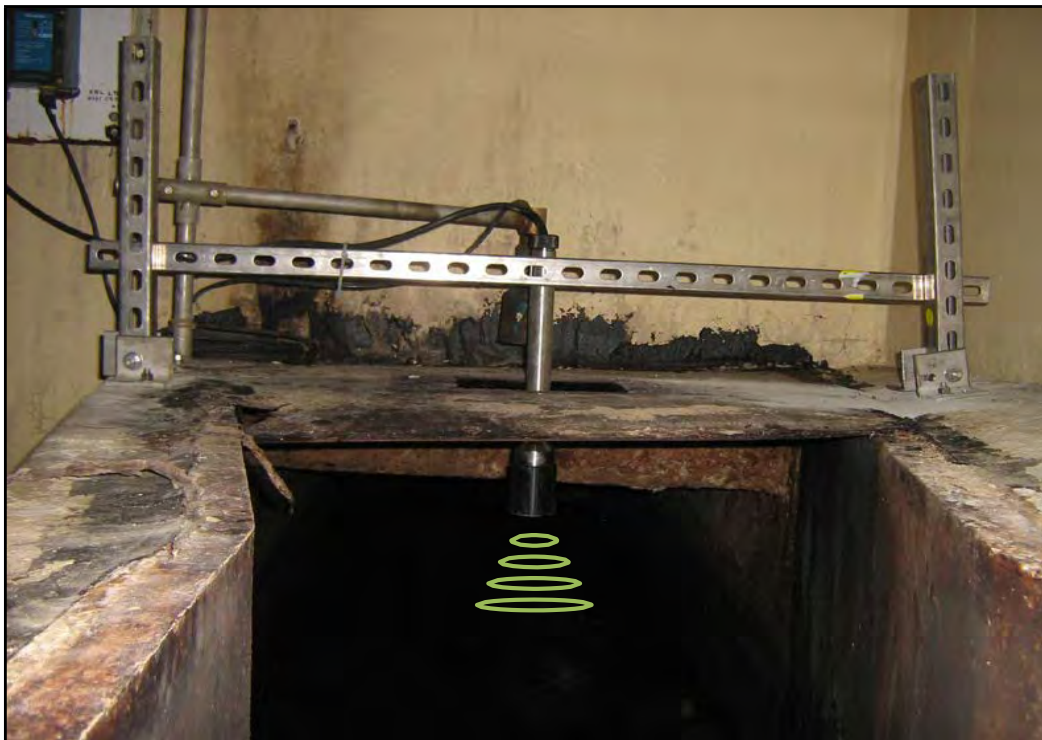
Figure 5. Parshall Flume Sensor Installation
