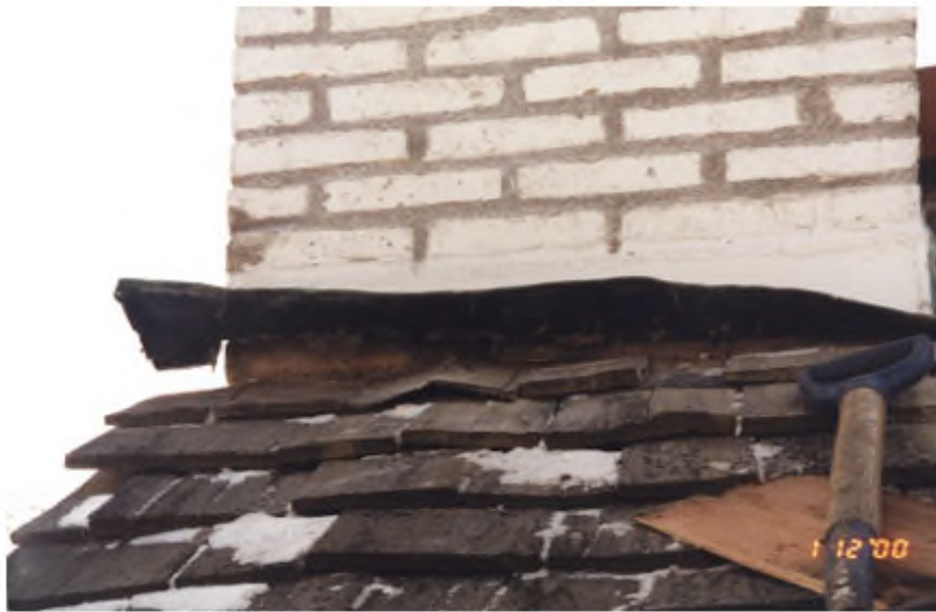
Apron flashing installed at a chimney on the roof systems north slope.
